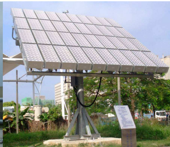
5kW Ground Mounted HCPV – NCKU, Tainan, Taiwan
